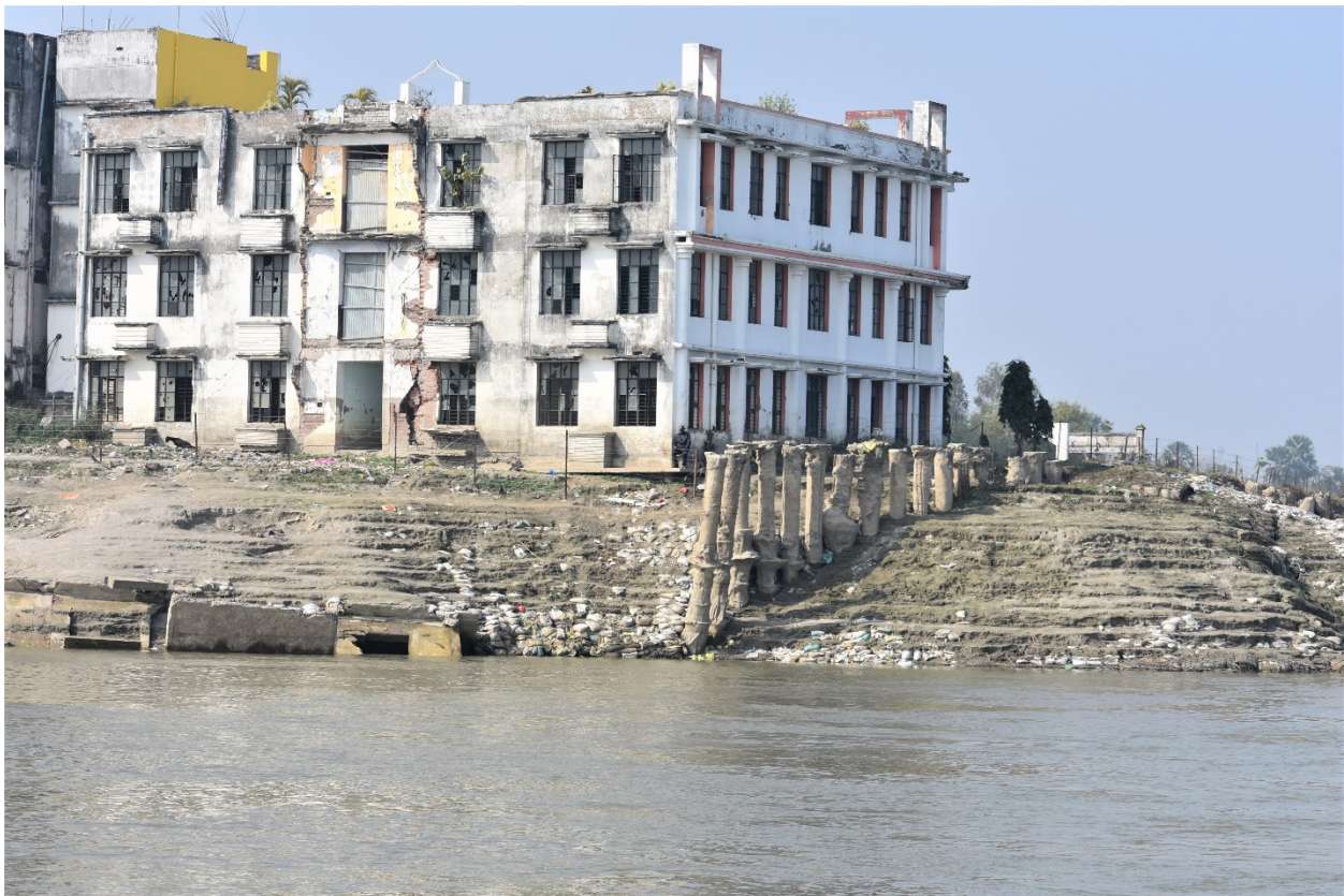
Image 38 : Part Of A School Complex Damaged Near Farka Facing Toe Erosion
