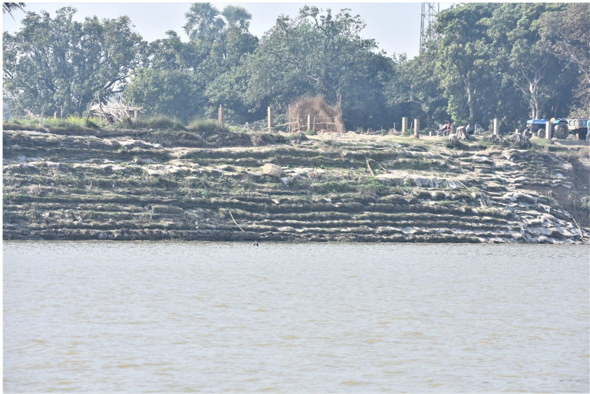
Image 40 : Erosion Control With Geotubes Along Ganga River Bank Near Sabour – Could be Durably and Economically Controlled by Riparian Grasses
