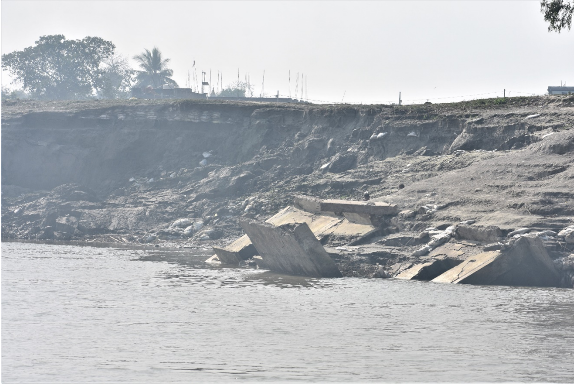
Image 39 : Destruction Caused By Erosion Between Sabour And Farka
